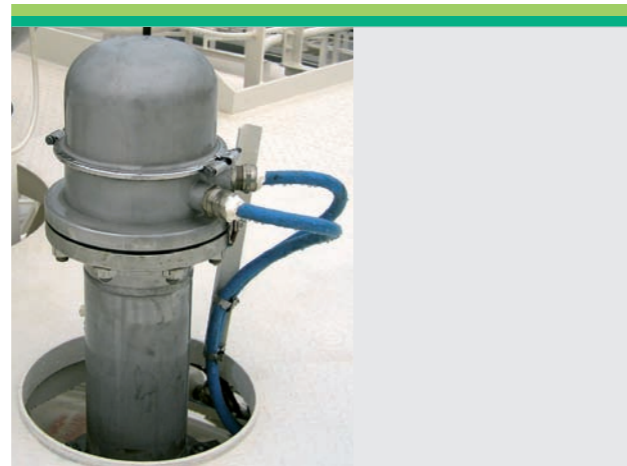
The OTG, Overfill Tank Gauge
