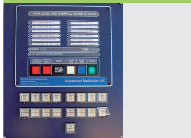
The OPA, Overfill Alarm Panel
