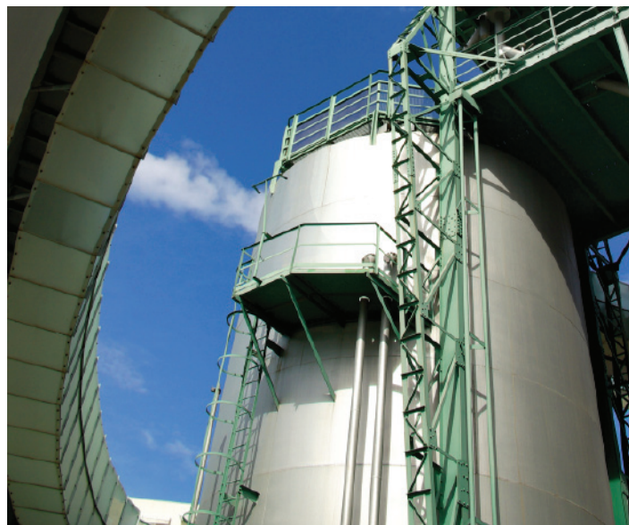
Gas bottling plant
