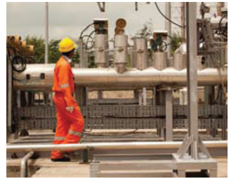
Figure 5: Cairn India Limited chose to install Daniel's fully engineered, integrated and pre-packaged custody transfer metering skids with ultrasonic accounting flow meters at each terminal along the Mangala pipeline.
