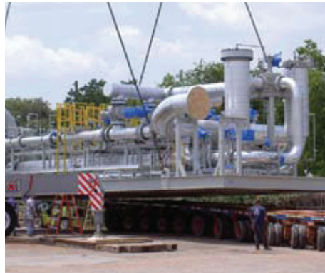
Figure 4: This photo illustrates the magnitude of a full-scale pipeline system. When such a metering system is handling between $5 million and $10 million worth of natural gas a day, flow measurement accuracy and repeatability become paramount.
